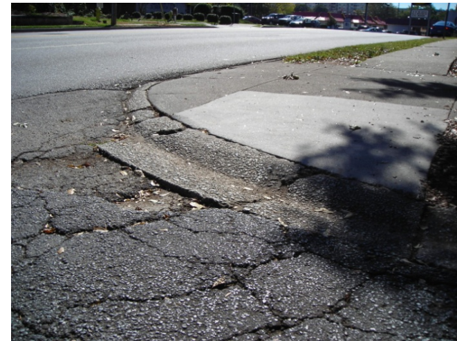
Patchy sidewalks and poorly maintained curb ramps make it difficult for those in wheelchairs to safely navigate the built environment
